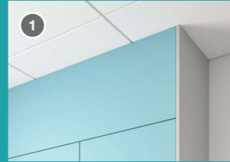
1 Ceiling infill panels stop unhygienic storage
